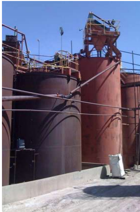
94,000 gal. total capacity primary leaching tanks and 56,000 gal. total capacity carbon absorption tanks
